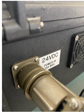
Figure 1: External Power Connection
